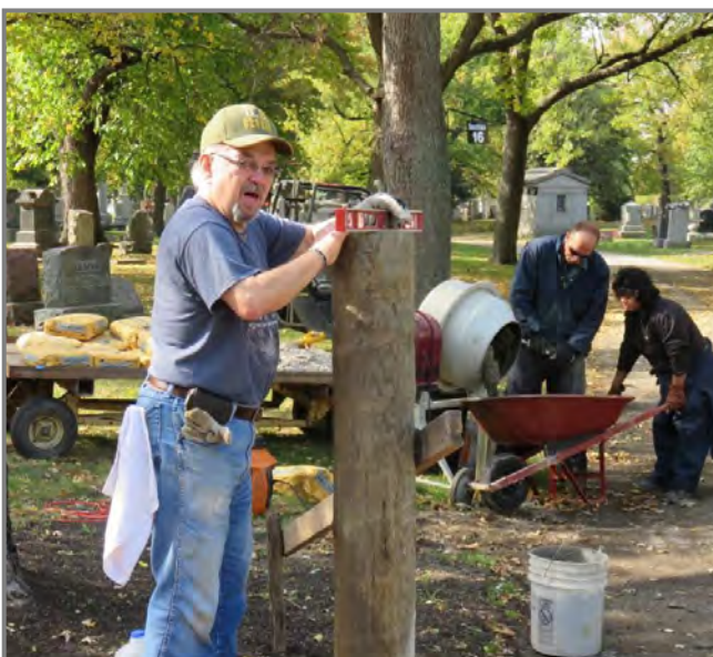
Jerry Gaydusek helping install the bollards at the Eastland Disaster Memorial at BNC.
